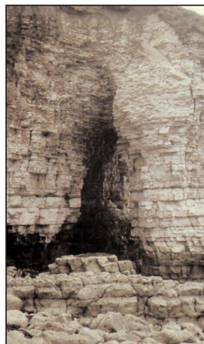
Figure 9: Taken only three months after the arch collapsed in 1984. Most of the debris has already disappeared
